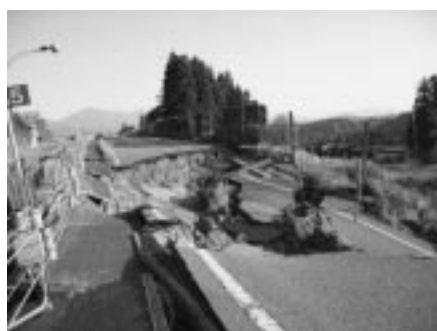
Chuetsu Earthquake (Collapsed lane on Kan-etsu Expressway) (Photograph: Japan Highway Public Corporation Hokuriku Branch)
